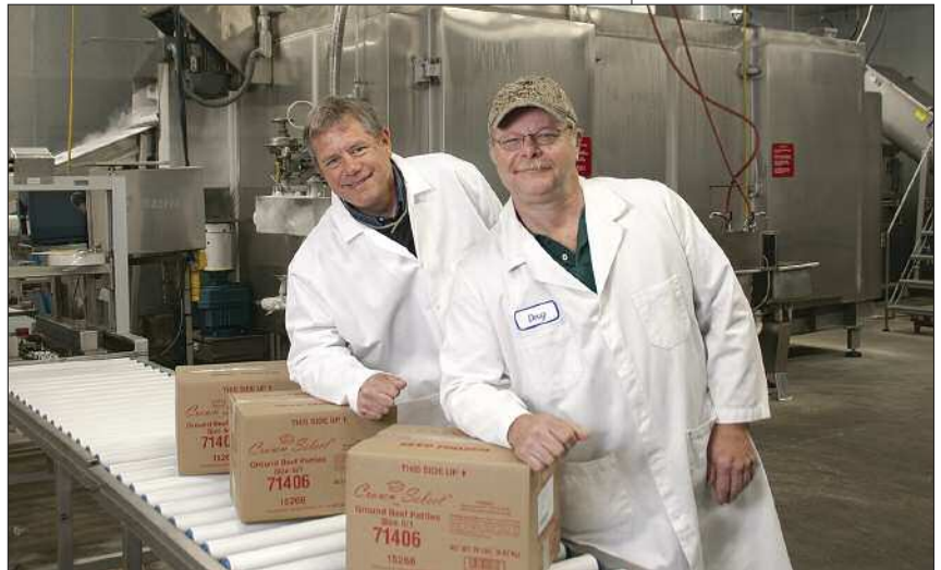
Ready to ship! John Jacobs, left, and Schenk’s Doug Richter lean on boxes of frozen hamburger patties that only minutes ago rolled off the conveyor of Schenk’s ultra performance spiral freezer, pictured behind them, at Schenk’s Mount Vernon, Wash., packing plant.
